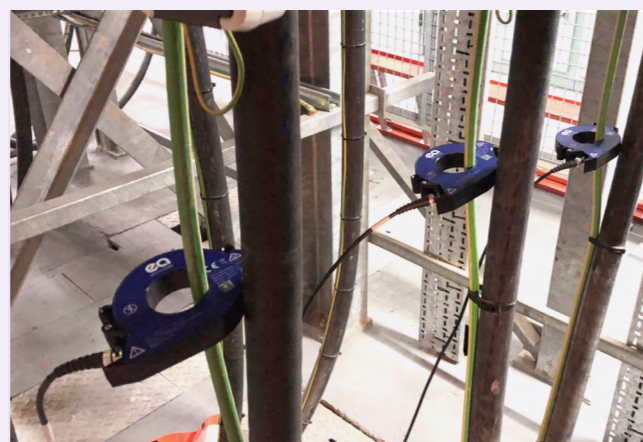
HFCT cable monitoring
